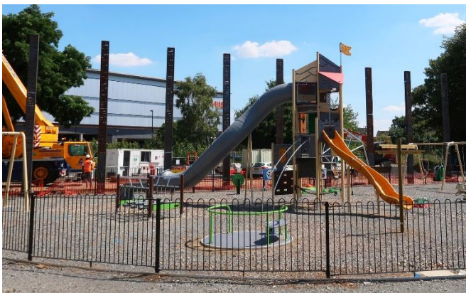
Castle Park under construction, showing the tall posts that hold the heritage storyboards
